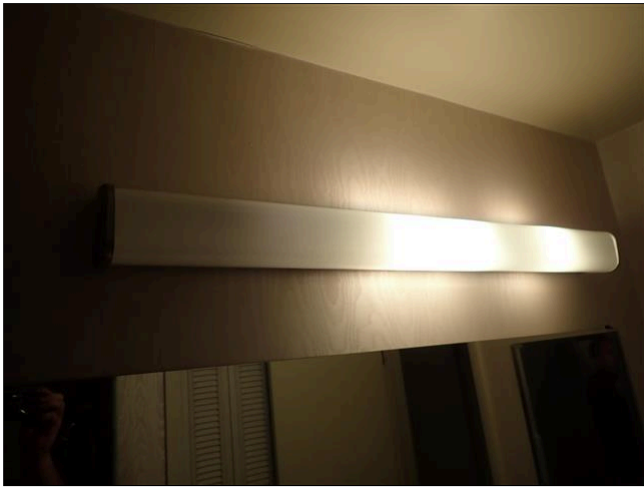
7.9(2) ELECTRIC / GFCI (Picture 1)
