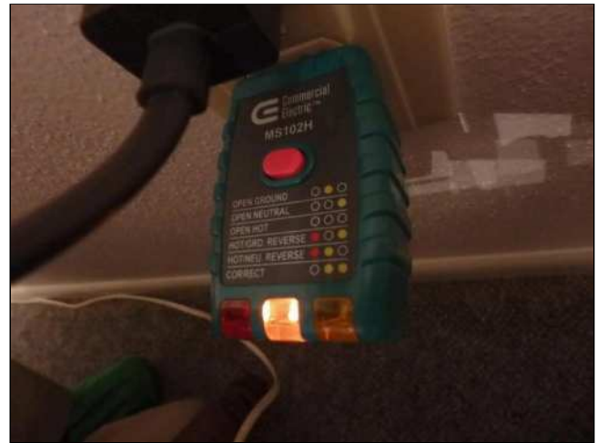
8.7(3) ELECTRIC / DEVICES (Picture 5)
