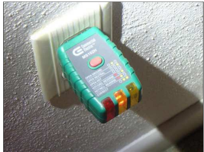
8.7(3) ELECTRIC / DEVICES (Picture 7)
