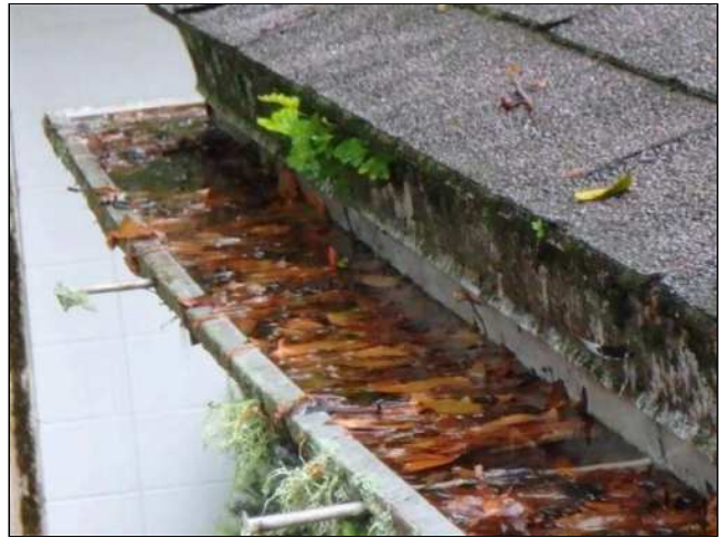
1.7(1) RAIN GUTTERS / EAVESTROUGHS (Picture 2)
