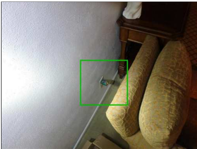
8.7(3) ELECTRIC / DEVICES (Picture 6)
