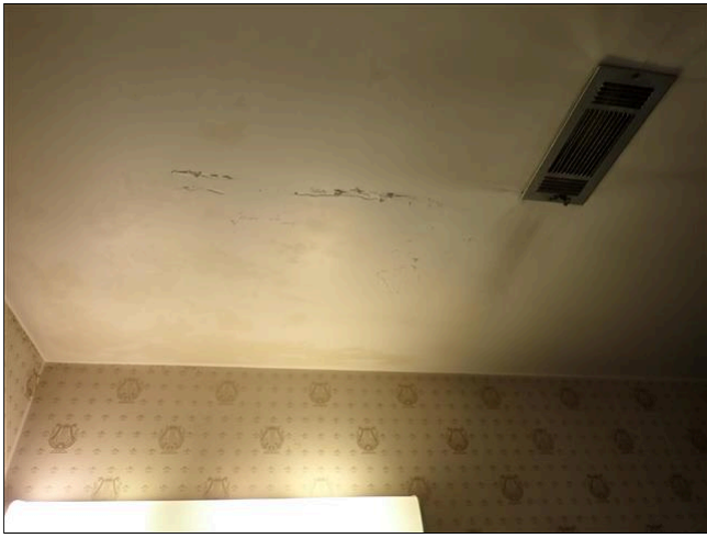
7.27(2) WALLS / CEILING (Picture 1)
