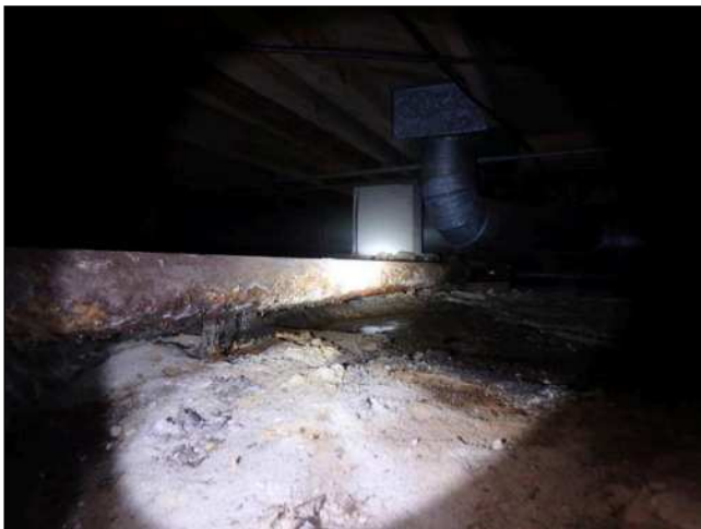
9.9(2) PLUMBING PROVISIONS (Picture 1)
