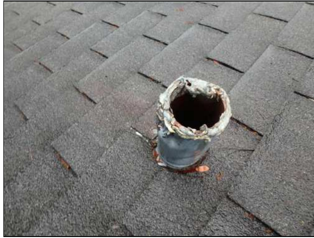
1.2 (2) CORROSION OBSERVED AT VENTILATOR COVER(S). Prolonged exposure to corrosion may result in premature wear / failure of affected components. Also note location of materials.
