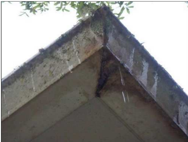
1.7(2) RAIN GUTTERS / EAVESTROUGHS (Picture 1)
