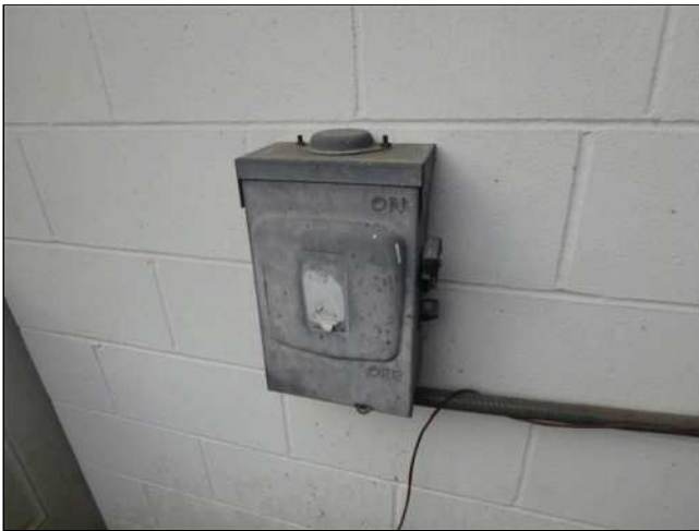
12.7 POWER / FUEL SOURCE (Picture 1)
