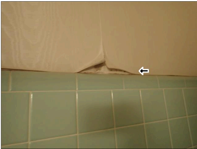
7.7 WALLS / CEILING (Picture 2)
