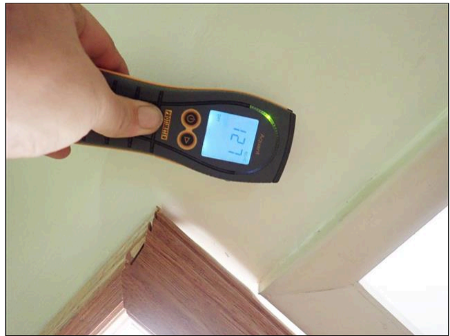
6.2 WALLS / CEILING (Picture 4)
