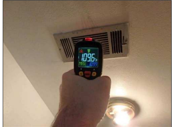
13.1(1) HEATING UNIT (Picture 2)
