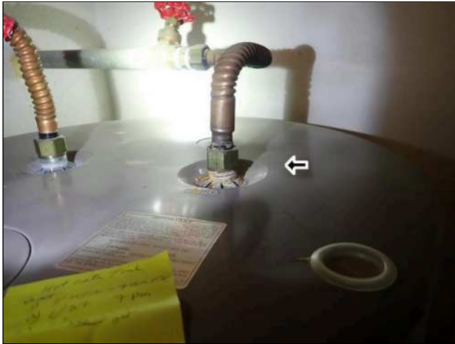
15.1(4) WATER HEATER (Picture 1)
