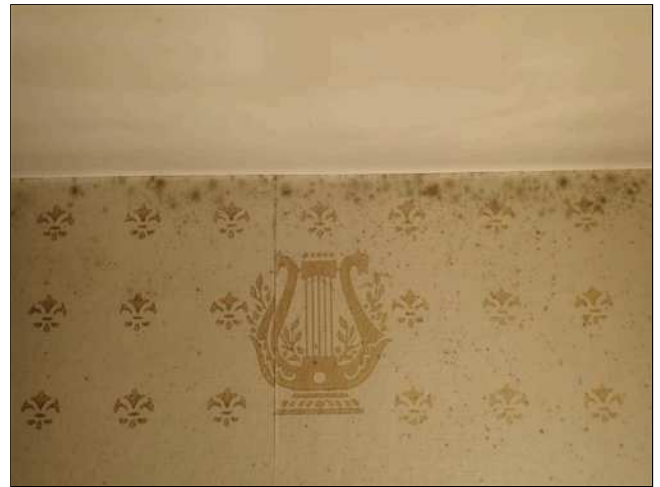
7.27(2) WALLS / CEILING (Picture 10)
