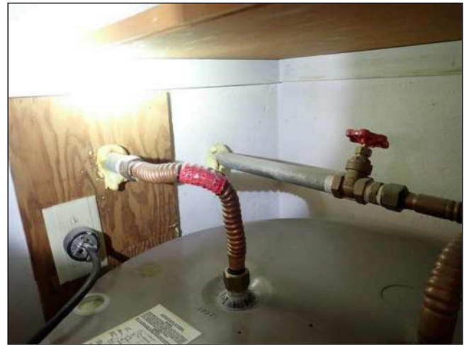
14.0(1) WATER SUPPLY PIPING (EXPOSED) (Picture 2)
