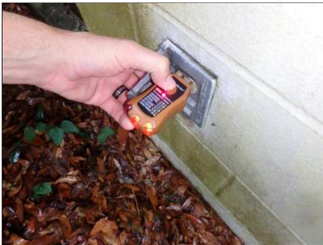
2.6(1) ELECTRIC / GFCI(S) (Picture 2)
