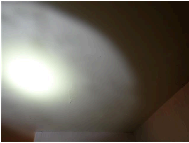
7.7 WALLS / CEILING (Picture 6)
