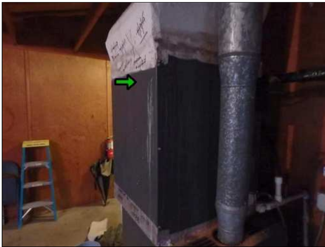
12.3 INDOOR UNIT (AIR HANDLER) (Picture 1)
