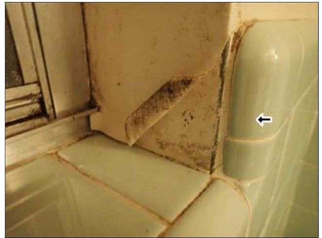
7.7 WALLS / CEILING (Picture 15)
