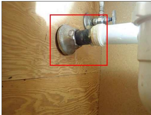
7.12 (3) CORROSION OBSERVED AT THE WATER SUPPLY SHUT-OFF VALVES AND/OR RELATED ELEMENTS. No leaks observed at time of inspection; however, prolonged exposure to corrosion may result in premature wear / failure of affected components. Removal of corrosion may result in exposure of leak. Condition of latent materials was not visible & could not be fully inspected. Hidden damage may exist.
