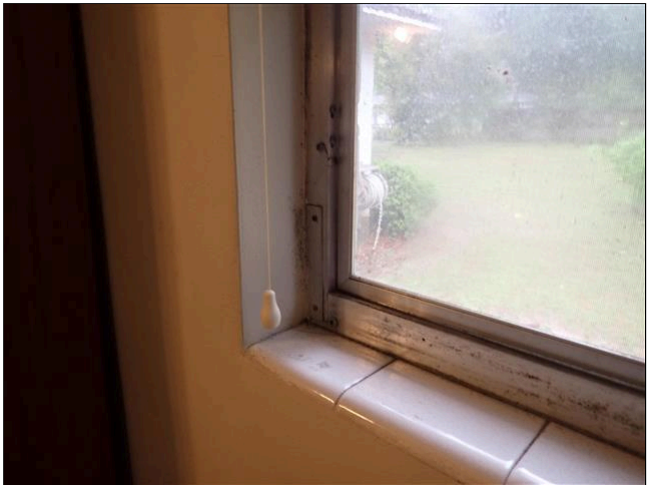
7.27(1) WALLS / CEILING (Picture 5)
