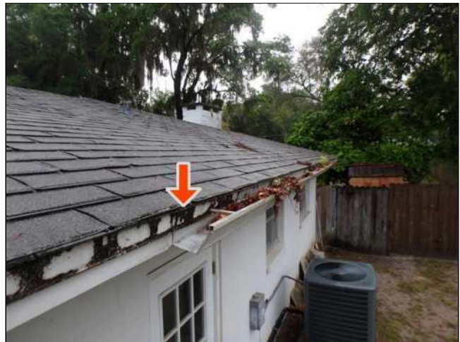
1.7(3) RAIN GUTTERS / EAVESTROUGHS (Picture 1)
