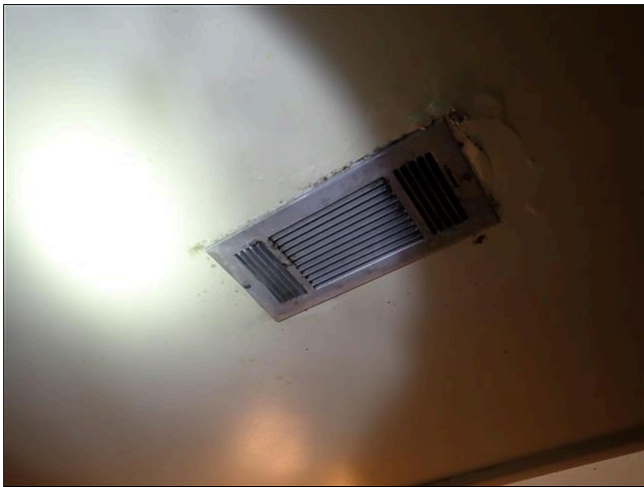
7.7 WALLS / CEILING (Picture 8)
