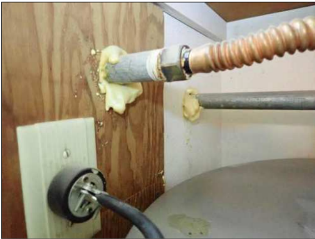
14.0(1) WATER SUPPLY PIPING (EXPOSED) (Picture 1)
