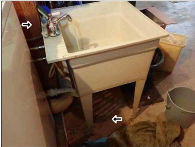
14.5(2) LAUNDRY SINK (Picture 1)
