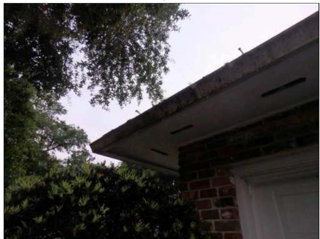
1.7(4) RAIN GUTTERS / EAVESTROUGHS (Picture 1)
