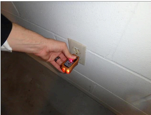
2.6(1) ELECTRIC / GFCI(S) (Picture 3)
