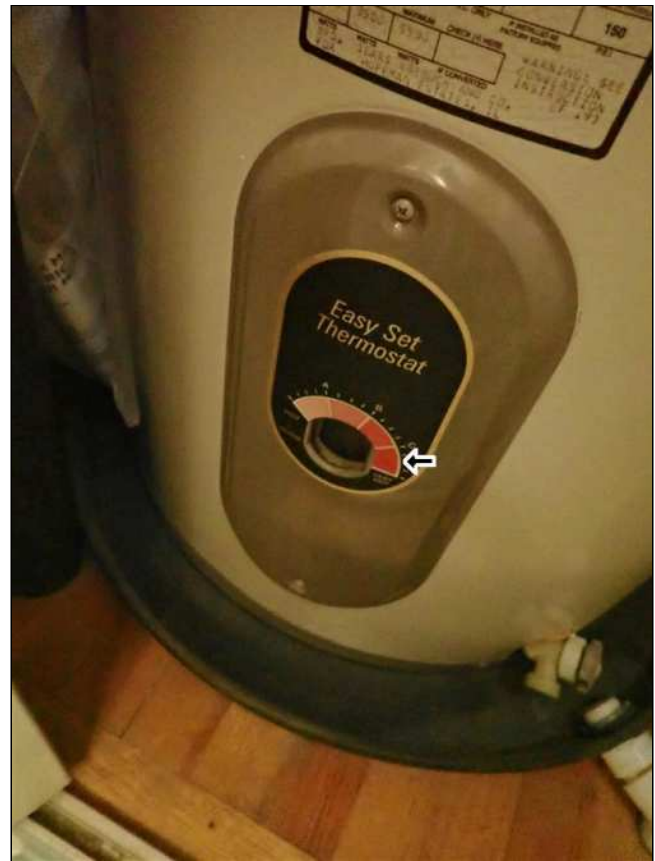
15.1(2) WATER HEATER (Picture 2)
