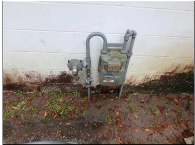
14.6(2) GAS PIPING (EXPOSED) (Picture 1)
