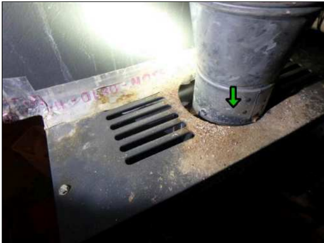
13.1(3) HEATING UNIT (Picture 1)
