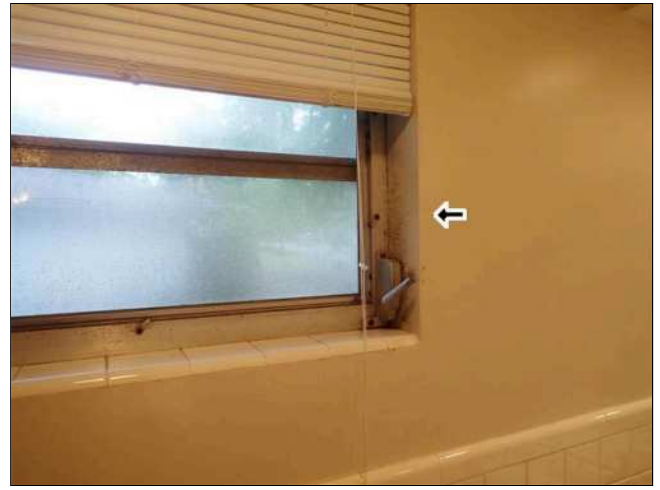
7.18 WALLS / CEILING (Picture 1)
