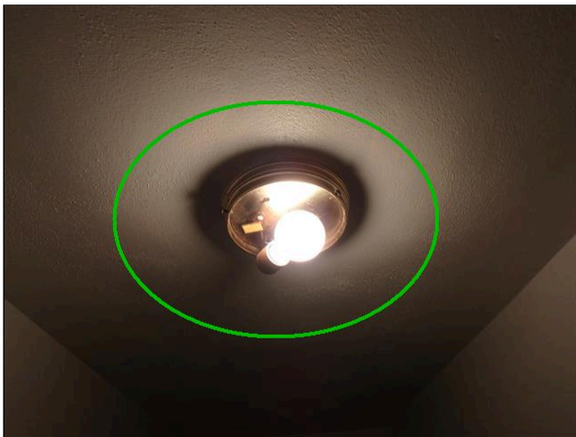
8.7(2) ELECTRIC / DEVICES (Picture 2)
