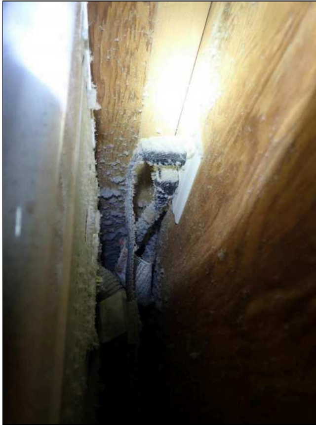
14.8 (2) DRYER LINT DISCHARGE TUBE / VENT COMPONENTS ARE DISCONNECTED - HOT AIR CAN BE FELT BEHIND DRYER WHEN UNIT IS RUNNING. Improper interface union may promote excessive lint accumulation which may pose a potential fire hazard.
