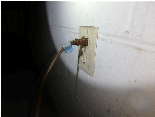
2.6(2) ELECTRIC / GFCI(S) (Picture 2)
