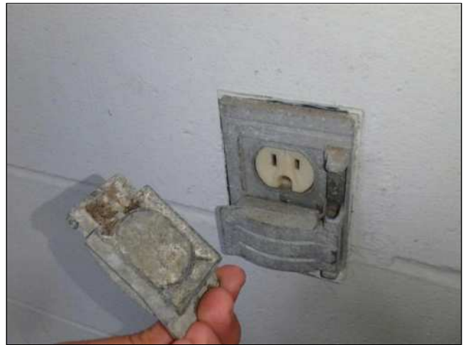
2.6(3) ELECTRIC / GFCI(S) (Picture 1)
