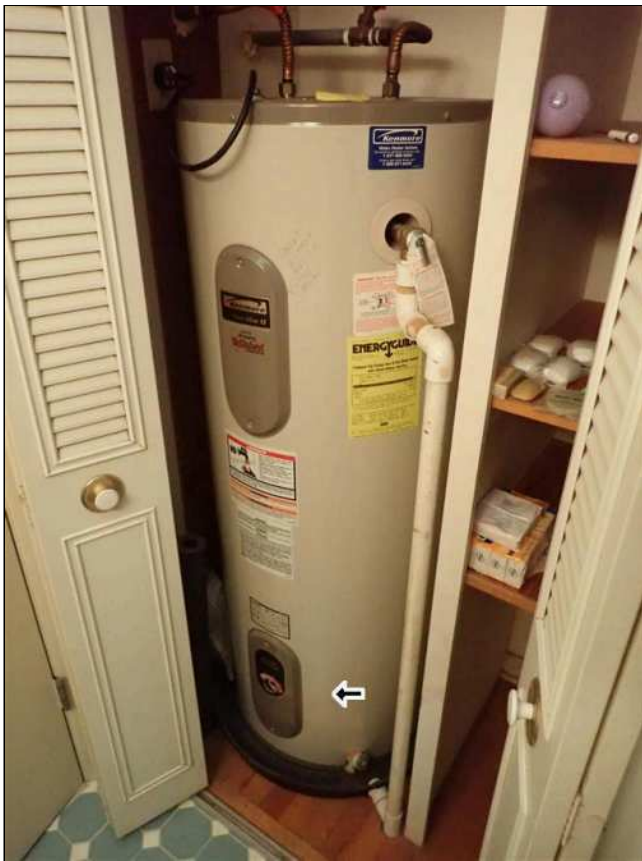
15.1(2) WATER HEATER (Picture 1)
