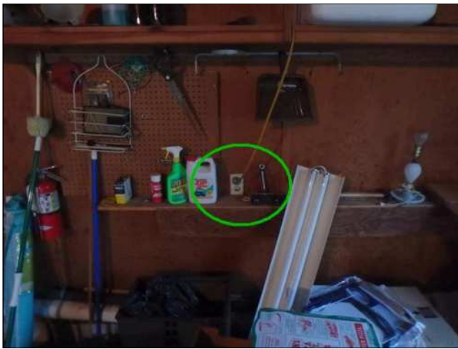
4.8 ELECTRIC / GFCI (Picture 1)
