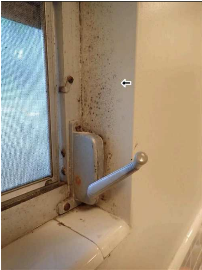
7.18 WALLS / CEILING (Picture 2)
