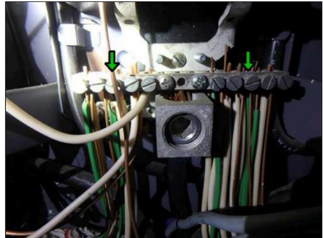
11.2(4) DISTRIBUTION PANEL (Picture 1)
