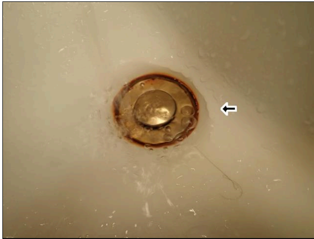
7.1 (4) HOT WATER PRESSURE IS POOR WHILE COLD WATER PRESSURE IS FAIR TO POOR. GALVANIZED WATER PIPING OBSERVED AT BATHROOMS AND KITCHEN. ALSO SEE PLUMBING COMMENTS. SUGGEST HAVING A LICENSED PLUMBER OR CONTRACTOR EVALUATE AND REPAIR OR REPLACE AS NEEDED.
