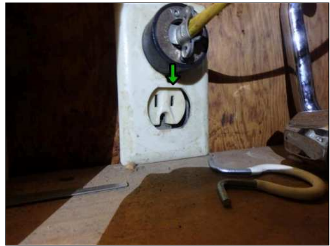
4.8 ELECTRIC / GFCI (Picture 2)
