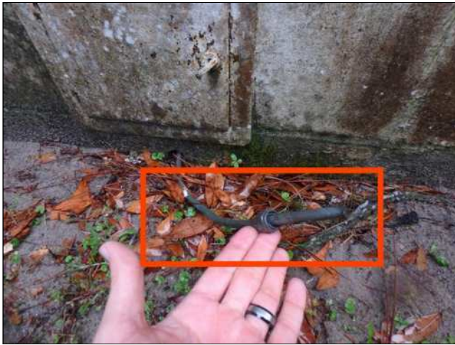
14.6(1) GAS PIPING (EXPOSED) (Picture 1)
