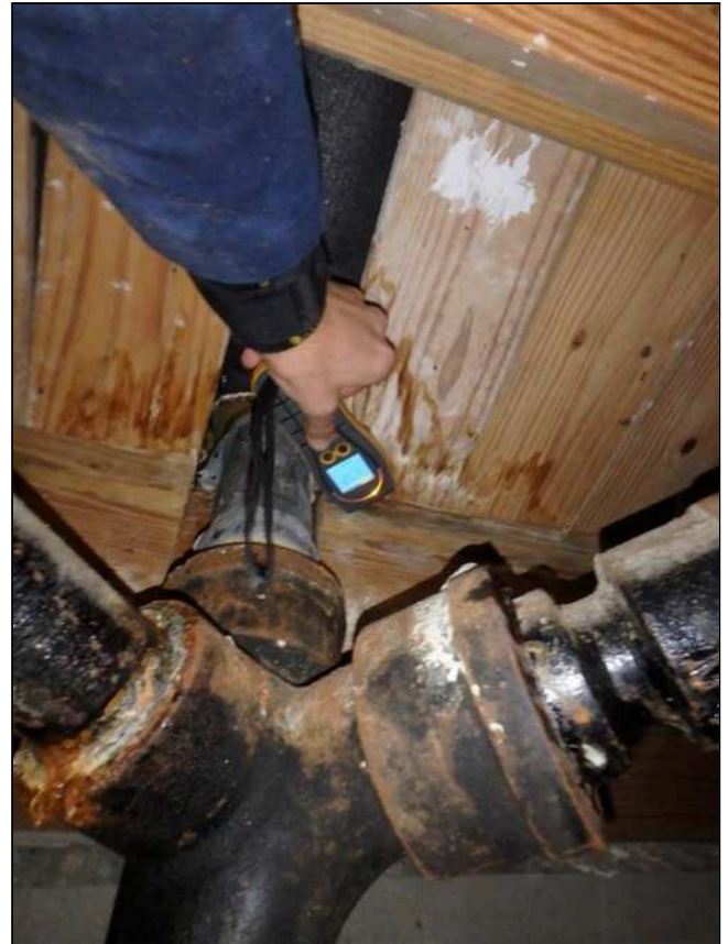
9.2 (3) STAINING & WOOD DECAY / DAMAGE OBSERVED AT THE SUB-FLOOR & FRAMING MATERIALS, MAINLY ADJACENT TO PLUMBING PROVISIONS. AREA(S) TESTED DRY USING A DIGITAL MOISTURE METER AT TIME OF INSPECTION. Wood decay / damage may deteriorate the integrity / rigidity of affected components over time. Condition of latent materials was not visible & could not be fully inspected. Hidden damage may exist.
