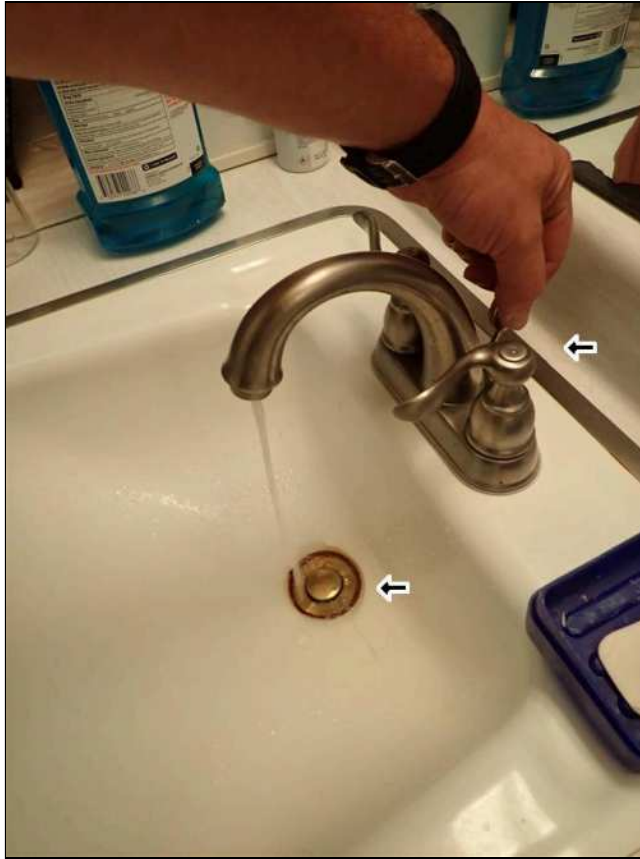
7.1 (3) RUST/CORROSION OBSERVED AT DRAIN OPENING AND DRAIN HARDWARE.
