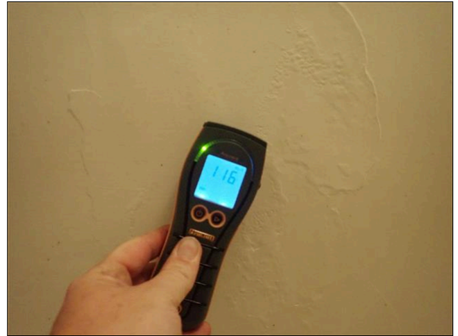
7.7 WALLS / CEILING (Picture 17)
