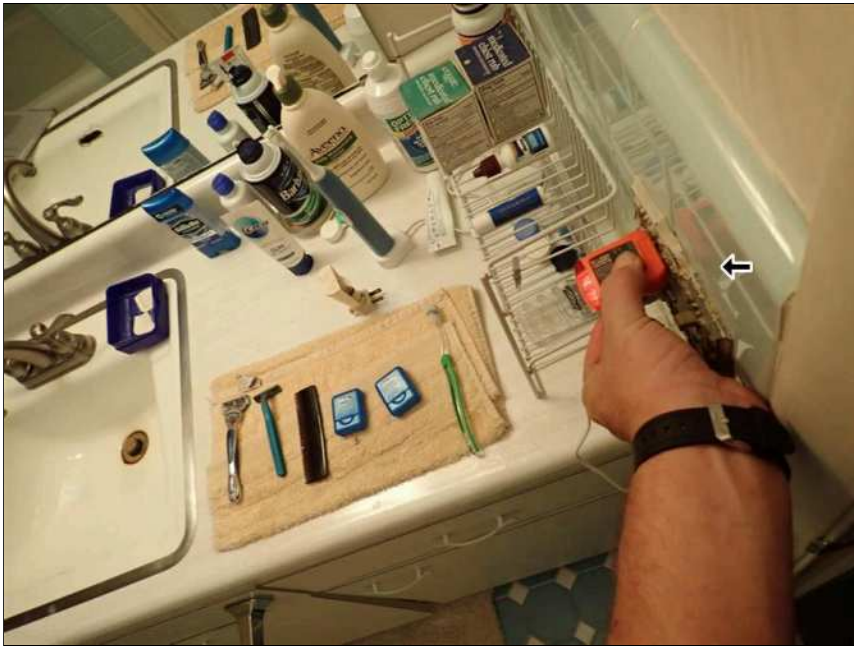
7.9(1) ELECTRIC / GFCI (Picture 1)
