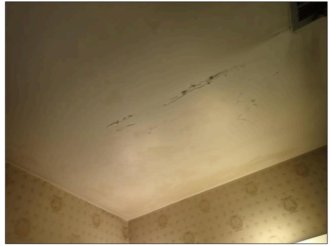
7.27(2) WALLS / CEILING (Picture 2)
