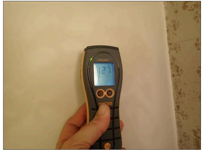
7.27(2) WALLS / CEILING (Picture 8)
