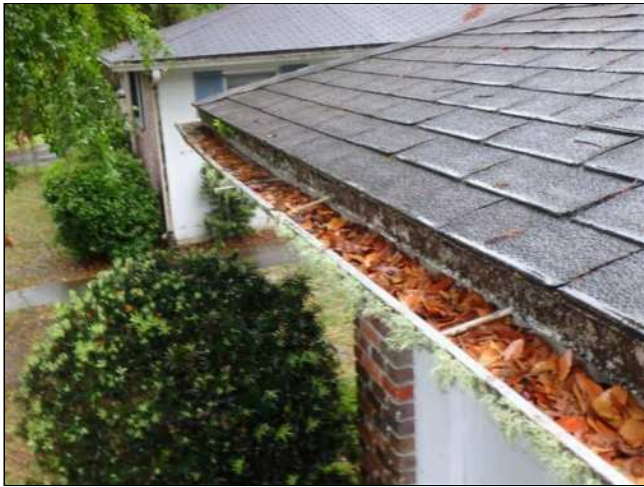
1.7(1) RAIN GUTTERS / EAVESTROUGHS (Picture 1)
