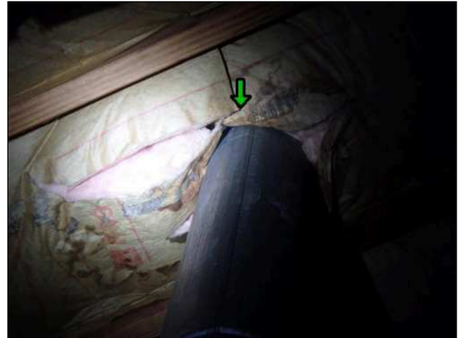
13.1(2) HEATING UNIT (Picture 2)
