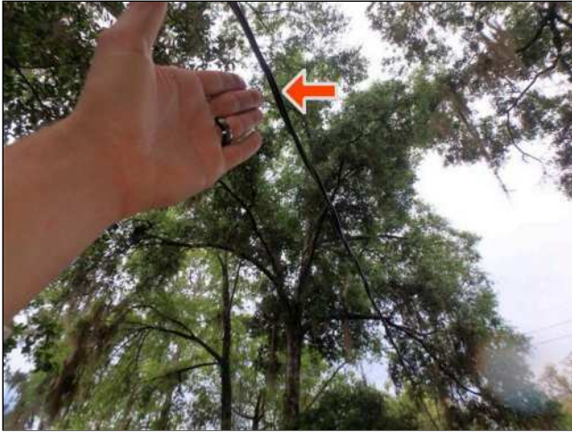
11.0(1) SERVICE / ENTRANCE LINE (Picture 1)
