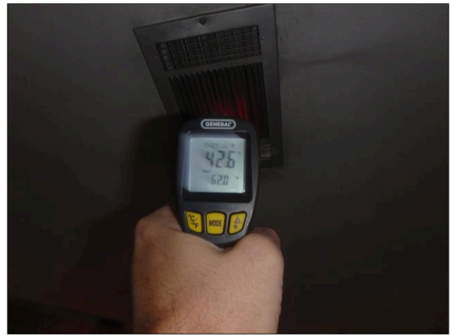
12.1(1) COOLING SYSTEM (Picture 2)
