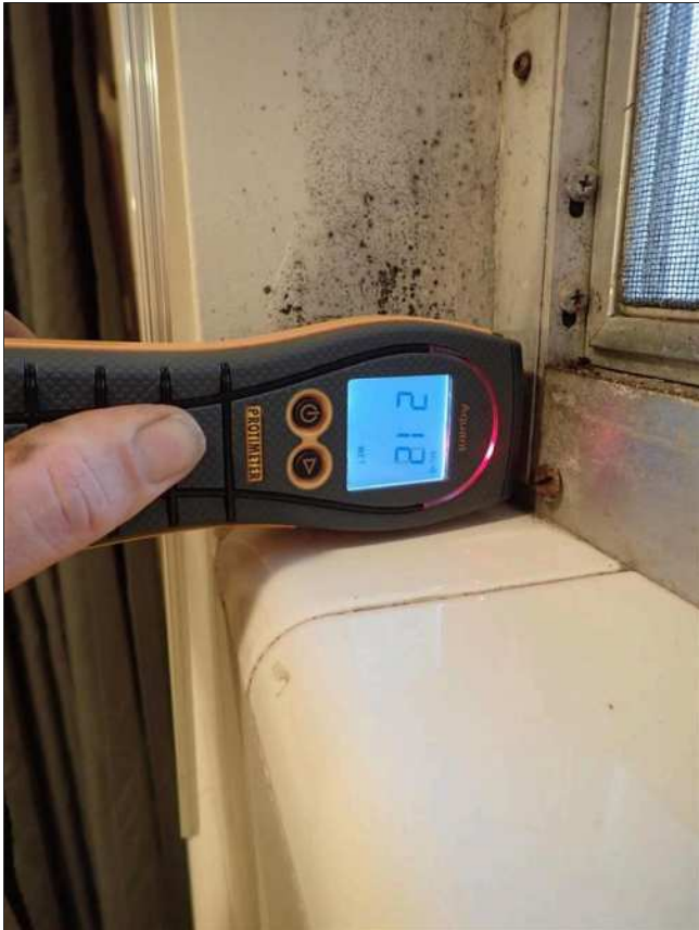
7.18 WALLS / CEILING (Picture 10)
