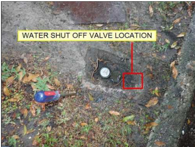
14.7(2) WATER METER (Picture 2)
