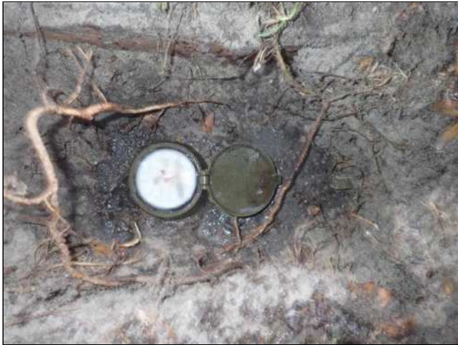
14.7(1) WATER METER (Picture 3)
