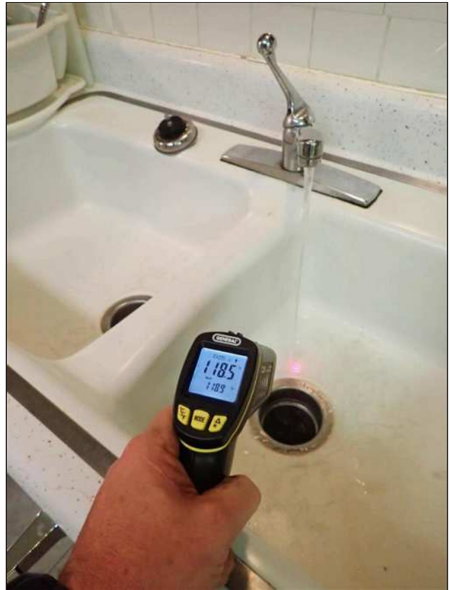
15.1(5) WATER HEATER (Picture 1)
