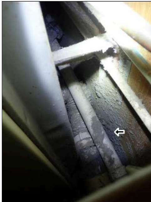
14.8 (3) EXTERIOR DRYER LINT DISCHARGE TUBE VENT COVER IS LOOSE / UNSECURED. Current condition may promote moisture / pest intrusion.
