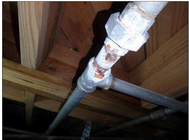
9.9(1) PLUMBING PROVISIONS (Picture 2)
