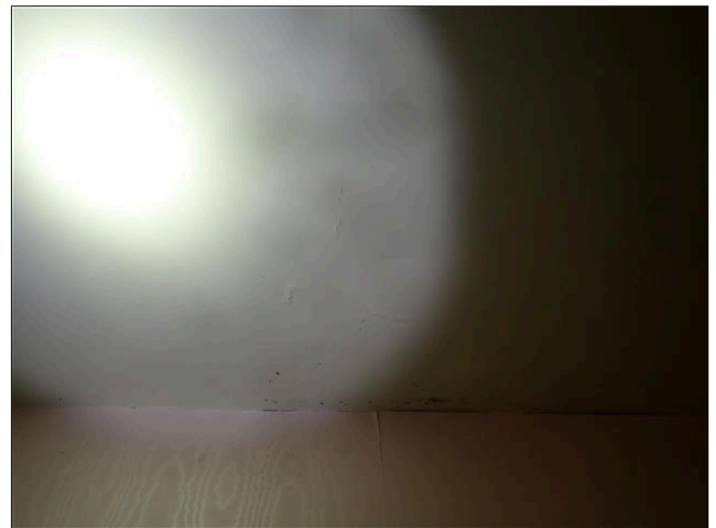
7.7 WALLS / CEILING (Picture 5)
