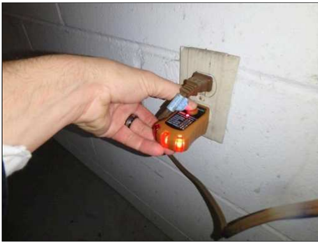
2.6(1) ELECTRIC / GFCI(S) (Picture 4)
