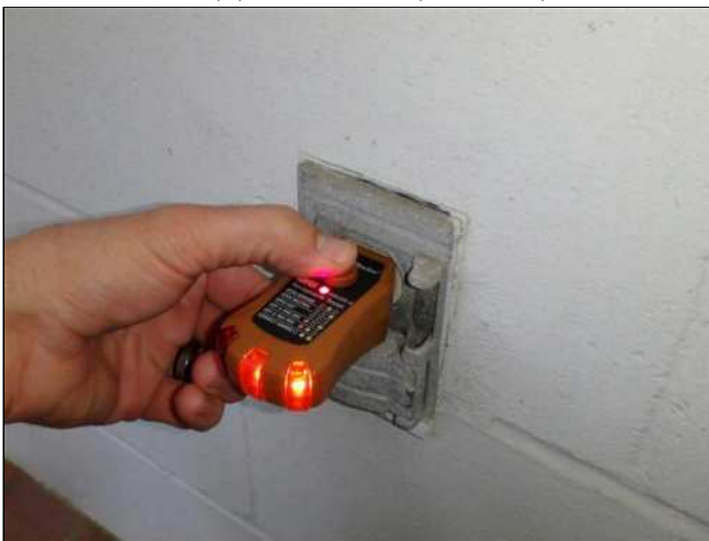
2.6(1) ELECTRIC / GFCI(S) (Picture 1)
