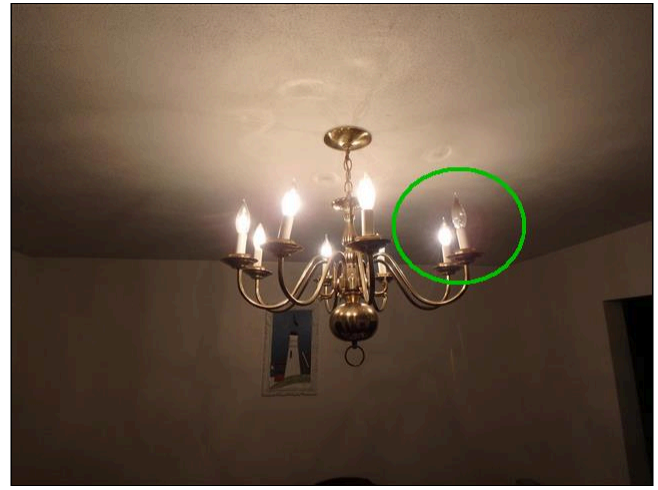
8.7(1) ELECTRIC / DEVICES (Picture 1)
