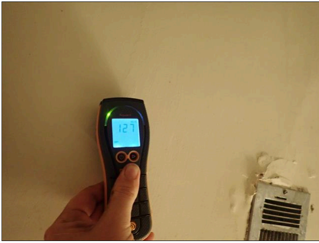
7.7 WALLS / CEILING (Picture 12)
