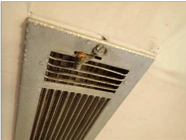
7.27(2) WALLS / CEILING (Picture 5)
