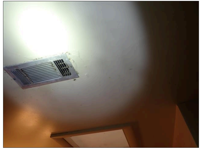
7.7 WALLS / CEILING (Picture 7)
