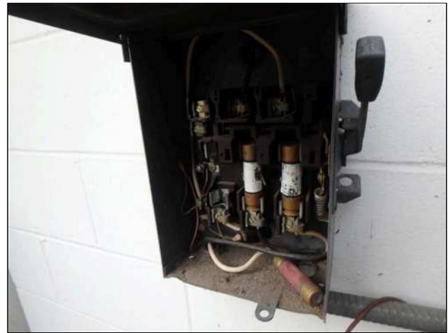
12.7 POWER / FUEL SOURCE (Picture 2)
