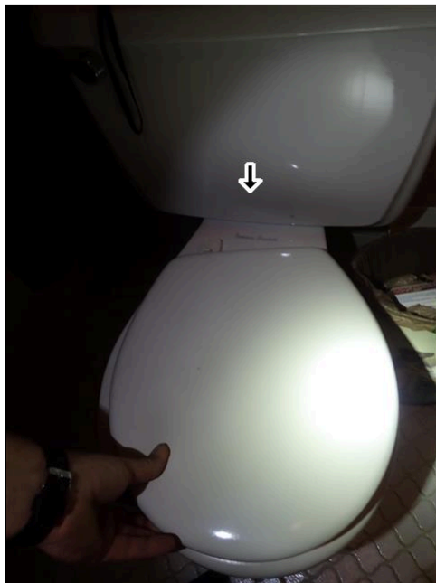
7.13 (5) TOILET IS LOOSE AT FLOOR AND MOVES SLIGHTLY WHEN STRADDLED.
