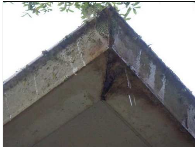
1.7 (3) MISSING END CAP(S) OBSERVED AT THE GUTTER SYSTEM. Missing end caps at gutters can cause erosion at the ground below the termination points. Many time the gutter has been installed to divert water away from an entryway. Erosion can often time be fixed with the addition of downspouts or other remedial methods such as gravel or swales.
