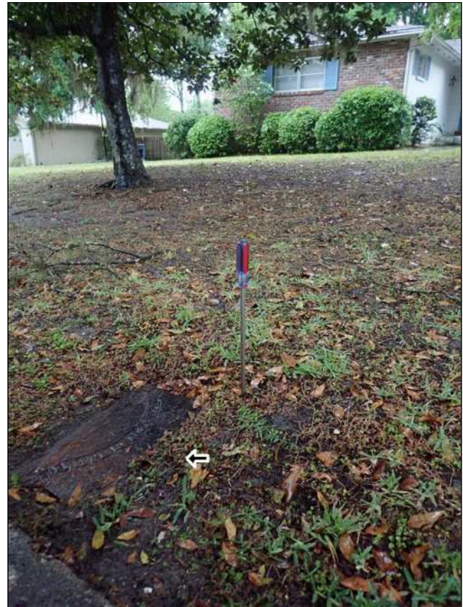
14.7(2) WATER METER (Picture 1)
