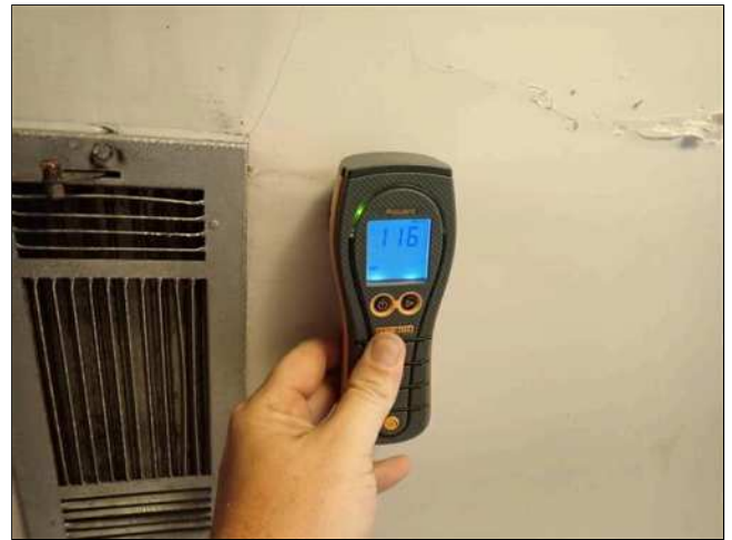
7.27(2) WALLS / CEILING (Picture 4)
