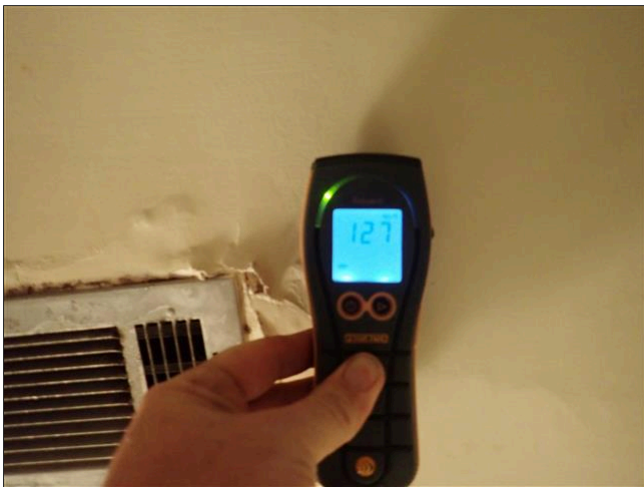
7.7 WALLS / CEILING (Picture 10)
