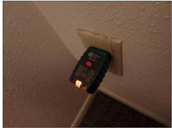
8.7(3) ELECTRIC / DEVICES (Picture 3)
