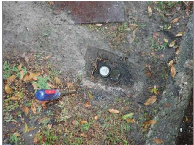
14.7(1) WATER METER (Picture 2)
